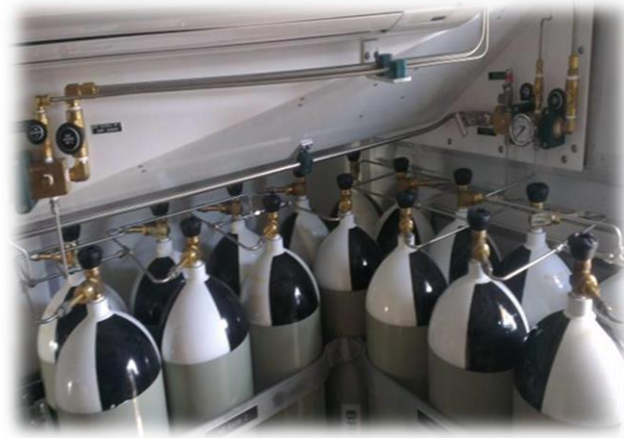
Cylinder Gas Bank
